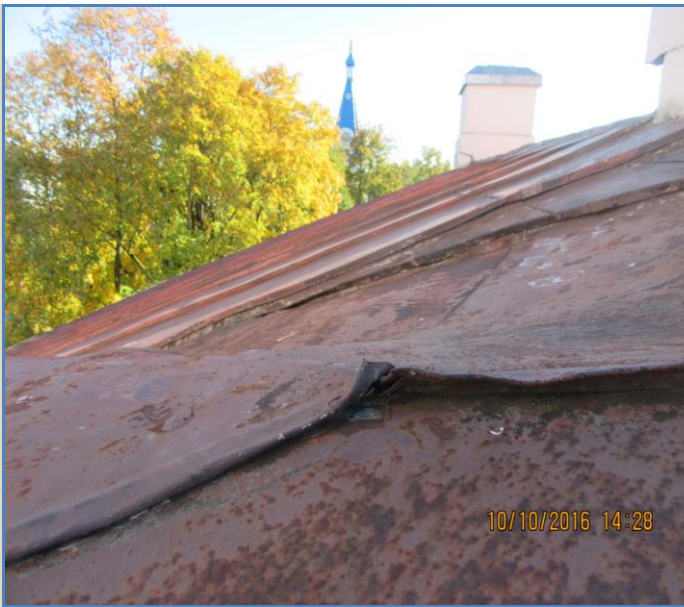
61.att.Jumta seguma defekts.
